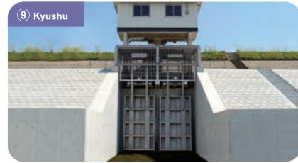
⑨ Kyushu Arase Sluice (2.00 m × 3.50 m, double) Orderer: Chikugogawa River Office, Kyushu Regional Development Bureau
