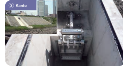
③ Kanto Futakotama Sluice (1.00 m × 1.00 m) Orderer: Kaihin River Office, Kanto Regional Development Bureau
