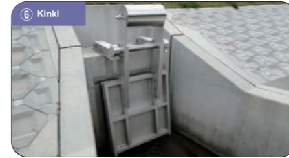
⑥ Kinki Noma River Drainage Sluice (1.60 m × 1.60 m) Orderer: Kitaharima Prefectural Bureau, Hyogo Prefecture
